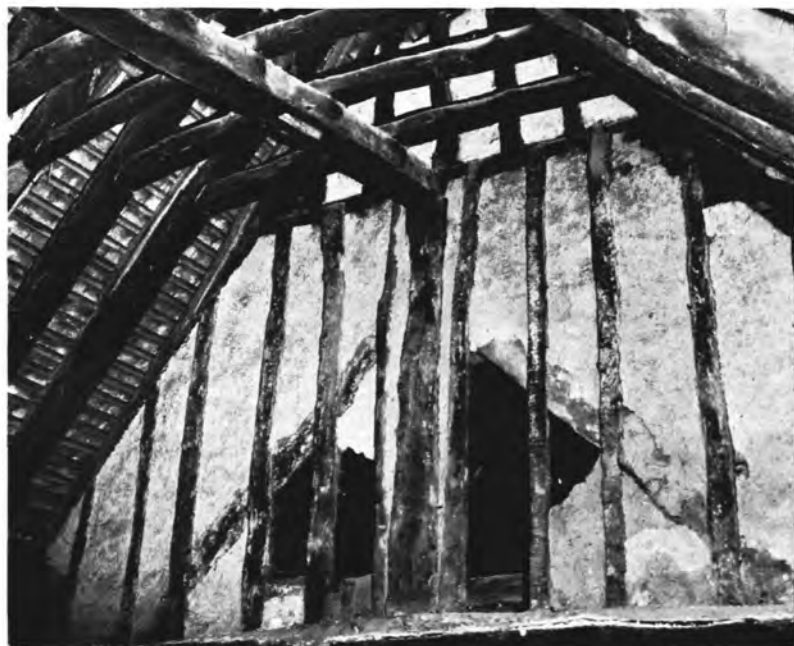
B. Upper part of North-west side of Partition between Hall and Room above Service.
