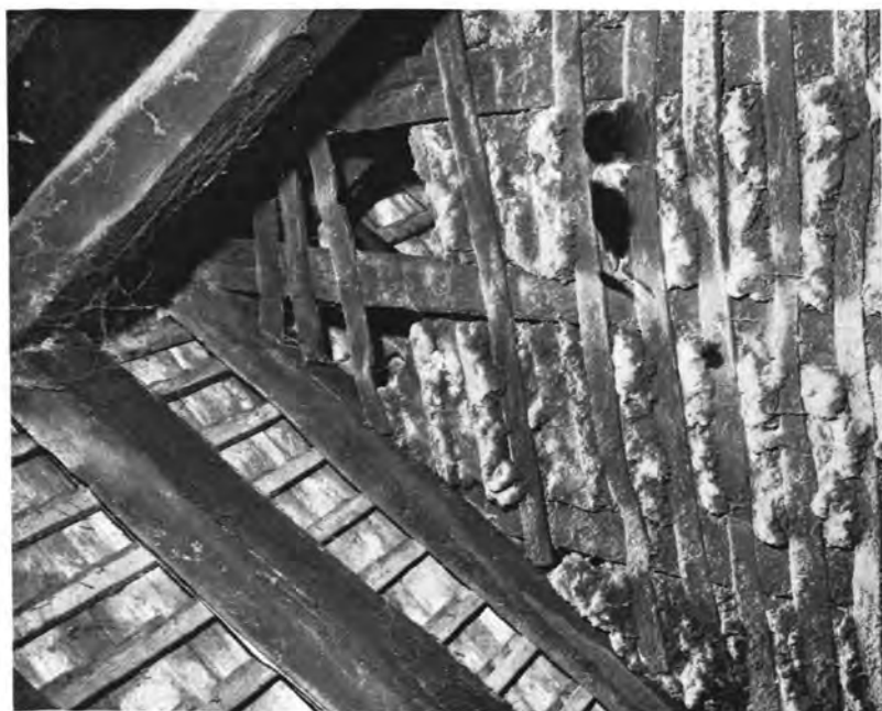
A. Space above Collar on line of Service Truss, showing Daub Filling unsmoothed towards Hall.
