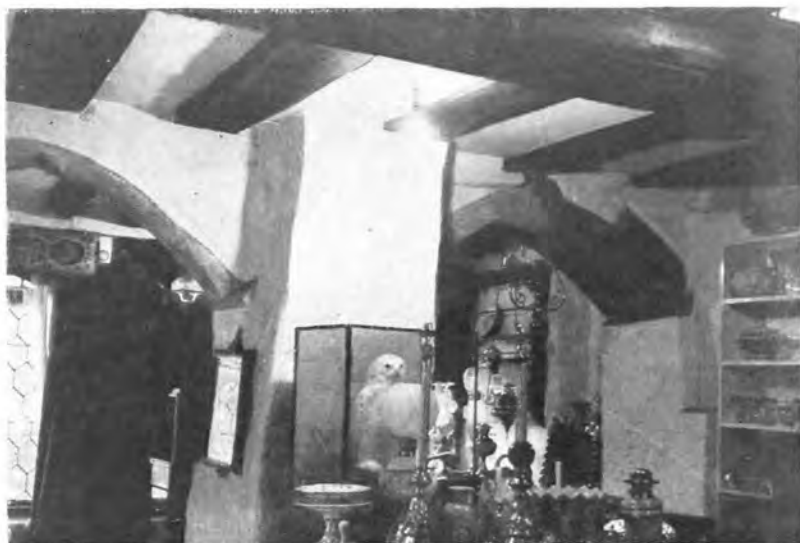
B. The massive Stone Pier and Arches, with original Joists at the Rear of the Shop.
