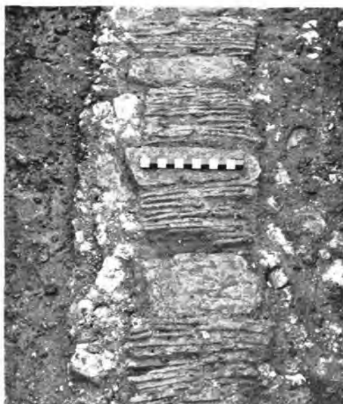
A. Reredorter drain, floored with stone slabs alternating with roof-tiles set on edge.
