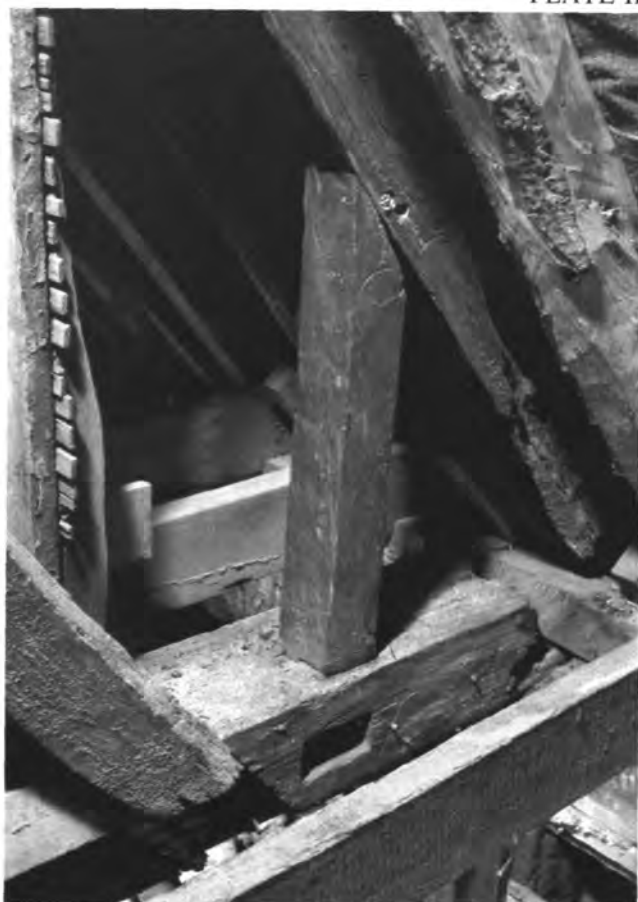
East end of central tie-beam, looking north showing cornice-plate mortice and ashlar piece
