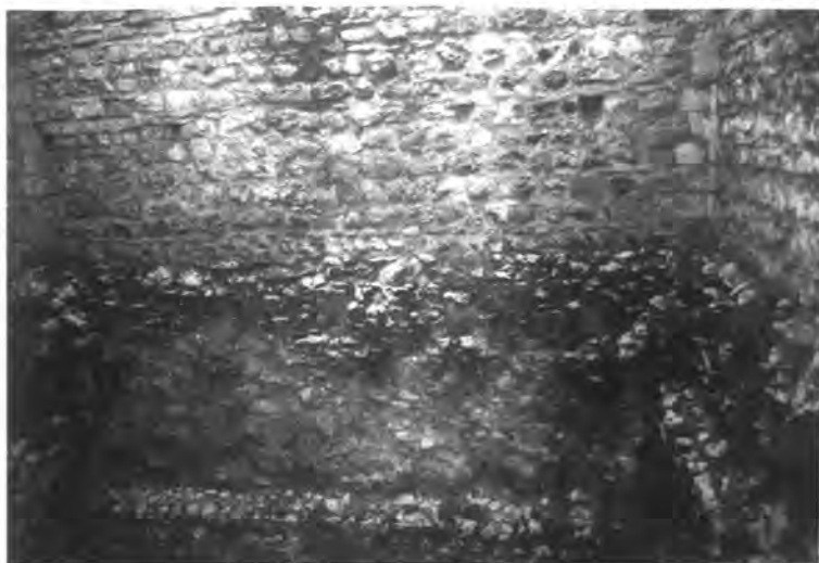
St Leonard's Tower: removed masonry at the internal offset level (south and west walls). Photograph: author
