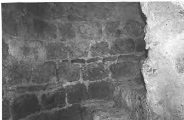
St Leonard's Tower: typical levelling courses in the vice wall. Photograph: author
